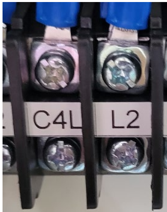
Pump POWER wires
