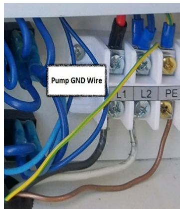
Pump GROUND wire.
